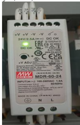
Gambar 5. Power Supply 24 VDC
