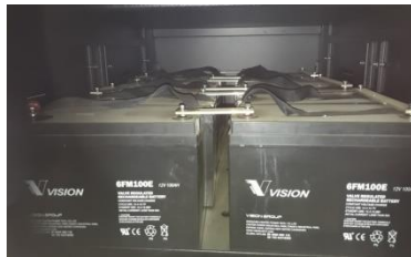
Gambar : Battery unit
