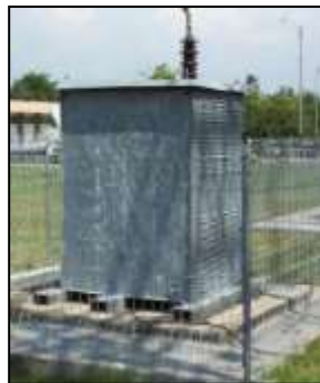
Gambar 1 Netral Grounding Resistor (NGR)
